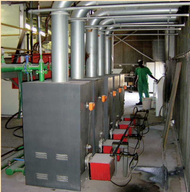
Oil stove to produce hot water or steam
